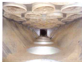
End inspection viewing panel.
